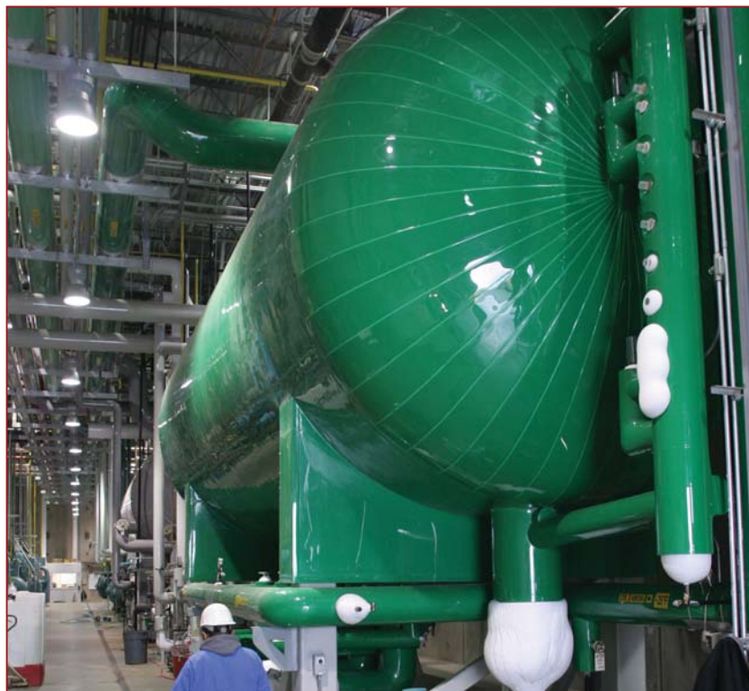
A 103,000-lb. capacity anhydrous ammonia storage tank stores liquid ammonia in Bakersfield’s flow-down refrigeration system. Photo by Alexander Horvath.
